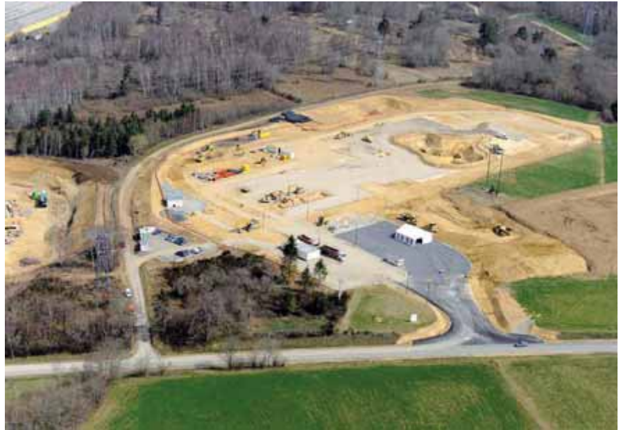
AERIAL VIEW OF THE UKAD CONSTRUCTION SITE AT SAINT-GEORGES DE MONS (FRANCE).
